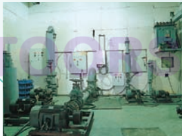
Testing area for Roots Blower
